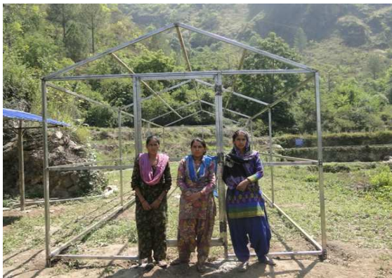
Structure of Poly house at Kapragad name tok, Bangdwara village – Photo on 01 st June 2017
