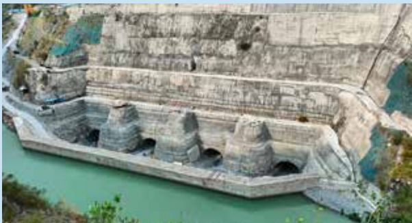
View of Concrete Lining in all limbs from the outer side of 1000 MW Tehri PSP
