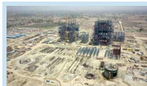
Aerial View of 1320 MW Khurja Super Thermal Power Project
