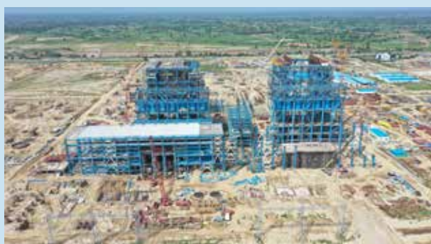
Erection of Boiler-1 & 2, MPH-1 & 2 and CCR Building in progress at 1320 MW KSTPP
