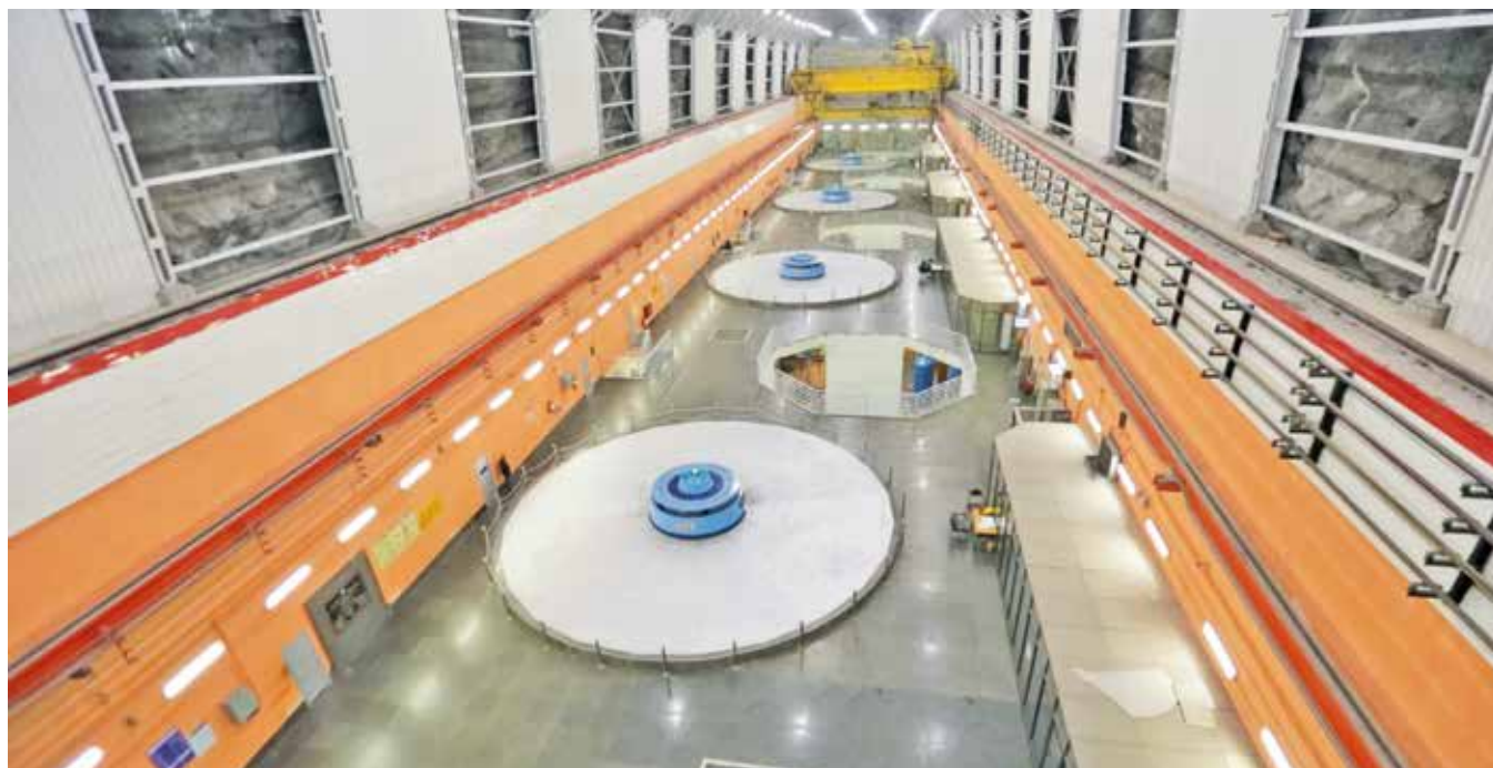
A view of Underground Power House of Tehri HPP(1000 MW)
