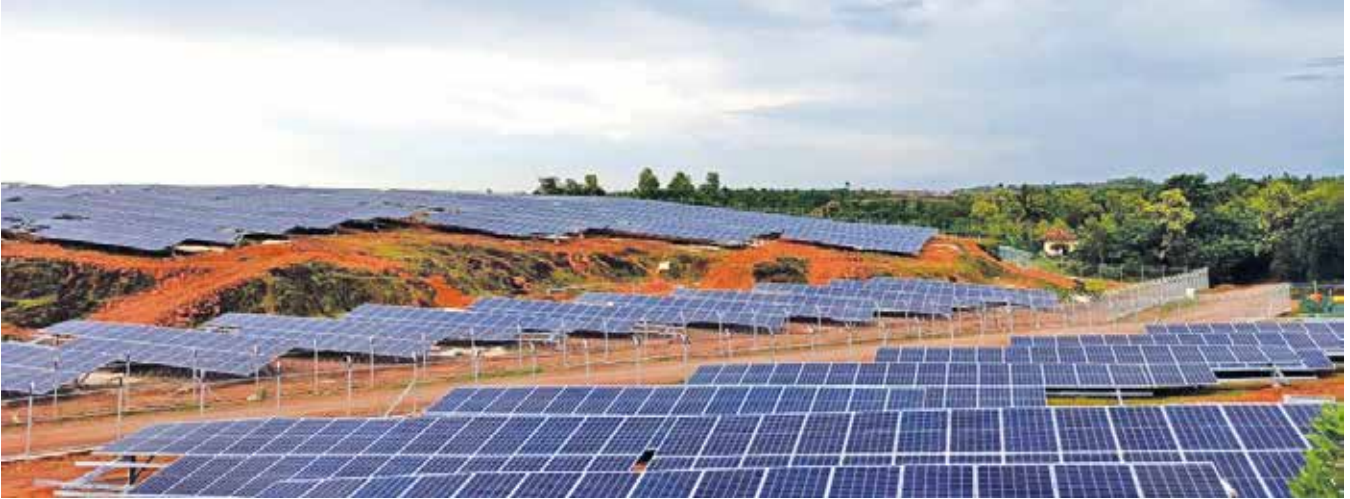
Installation of Solar Modules in advance stage at Solar Power Plant (50 MW), Kasargod, Kerala
