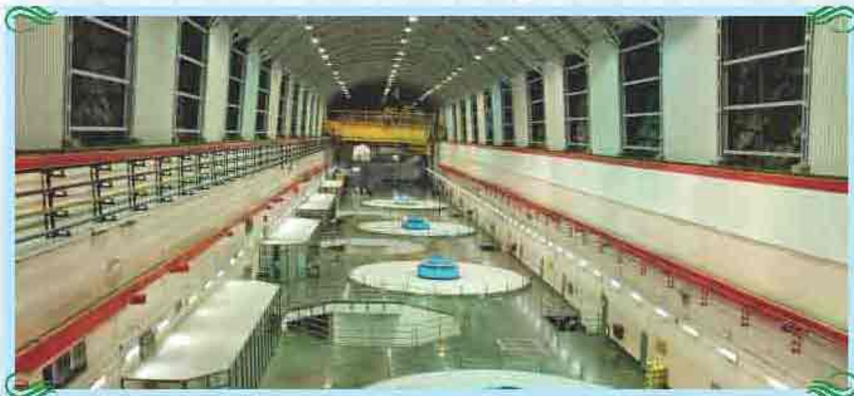
A view of Underground Power House of 1000 MW, Talmi HPP
