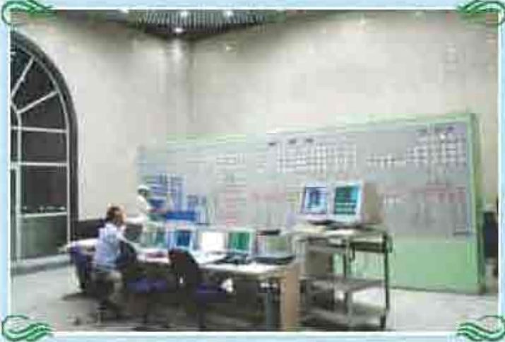
Computerised Control System of Underground Power House of Tehri HPP
