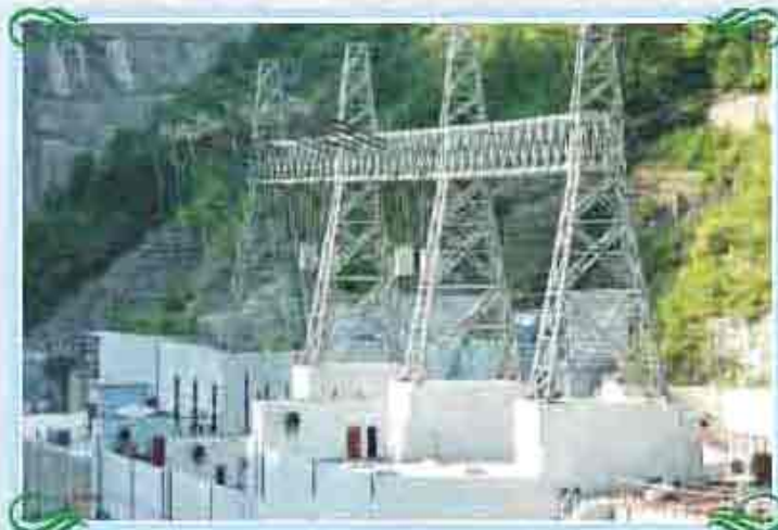
Power Evacuation from Tehri HPP
