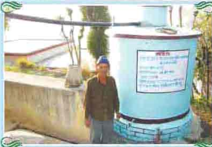
Rain Water Harvesting Tanks for water conservation at nearby Village of Tehri Dam Reservoir
