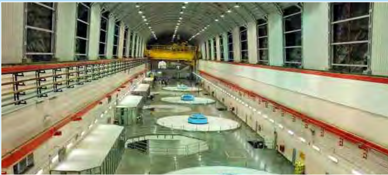
Under-ground Power House (1000 MW)
