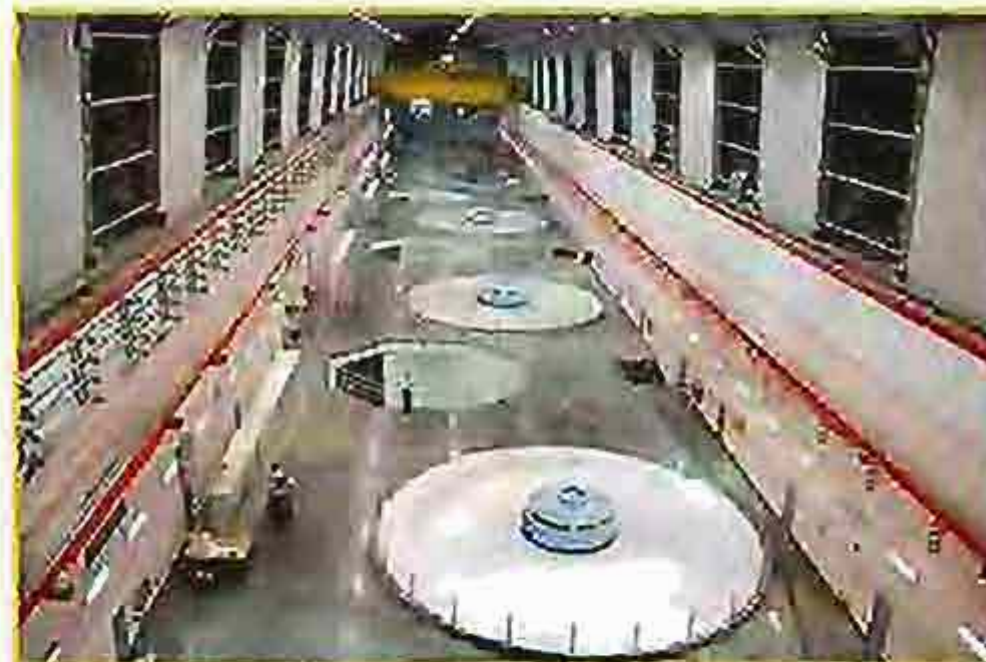
Under Ground Power House : Turbine / Generator Units in Machine Hall
